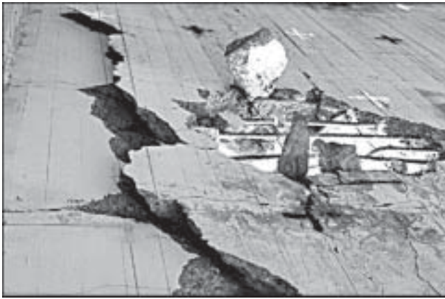
Fig 2 A typical punching shear failure of a bridge deck 4
